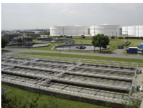
LRSA Primary Clarifiers
